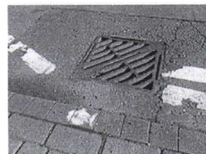
Blue drain and yellow fish symbol used by the UK Environment Agency to raise awareness of the ecological impacts of contaminating surface drainage.
