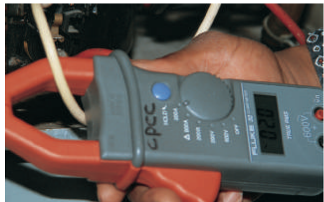
Figure 45-95 Taking a current reading at the compressor. Photo by Bill Johnson
