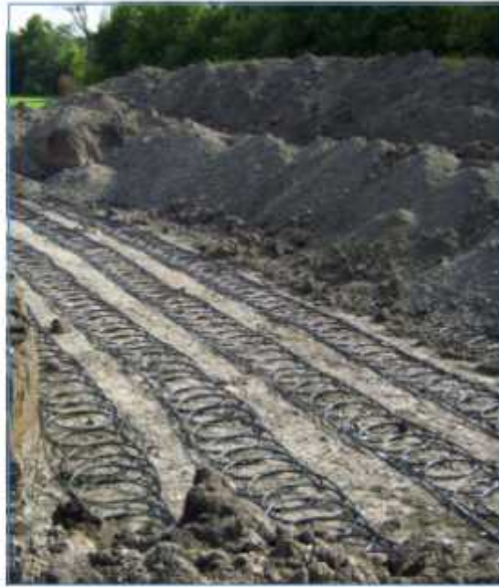
Figure 5. Horizontal ground loop (after)
