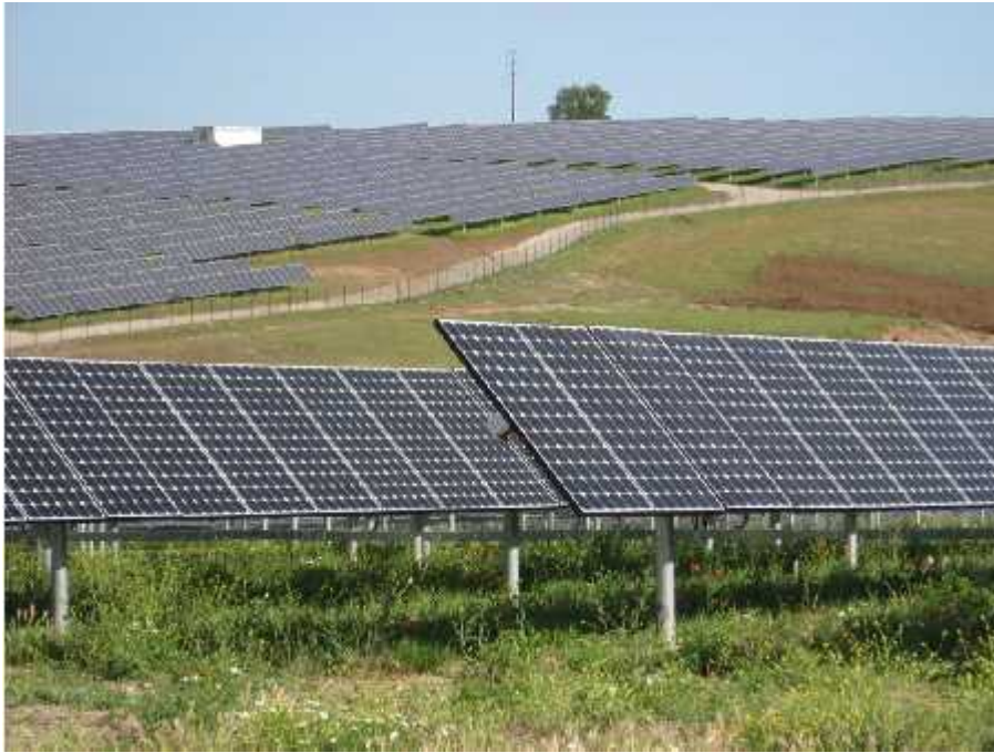
11 MW solar power plant near Serpa, Portugal
